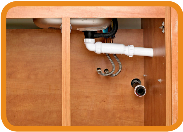
Domestic sink with waterless trap
